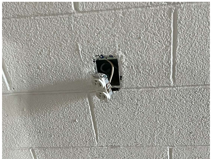
Figure 5. Broken Electrical Outlet
