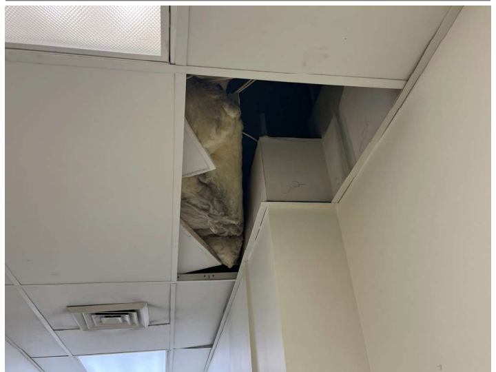
Figure 6. Missing Ceiling Tile
