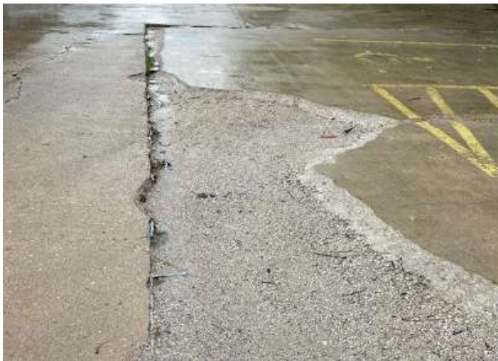
Figure 4. Concrete Cracks in Employee Parking Lot
