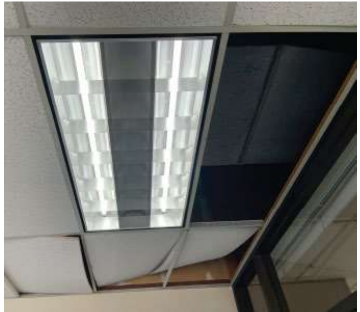
Figure 5. Missing Ceiling Tiles in Customer Lobby
